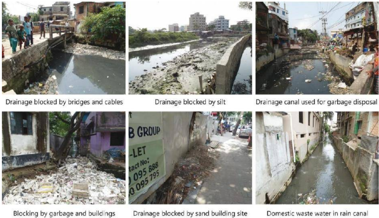
Figure 41 Images of blockages of drainage canals in Dhaka and Chittagong
